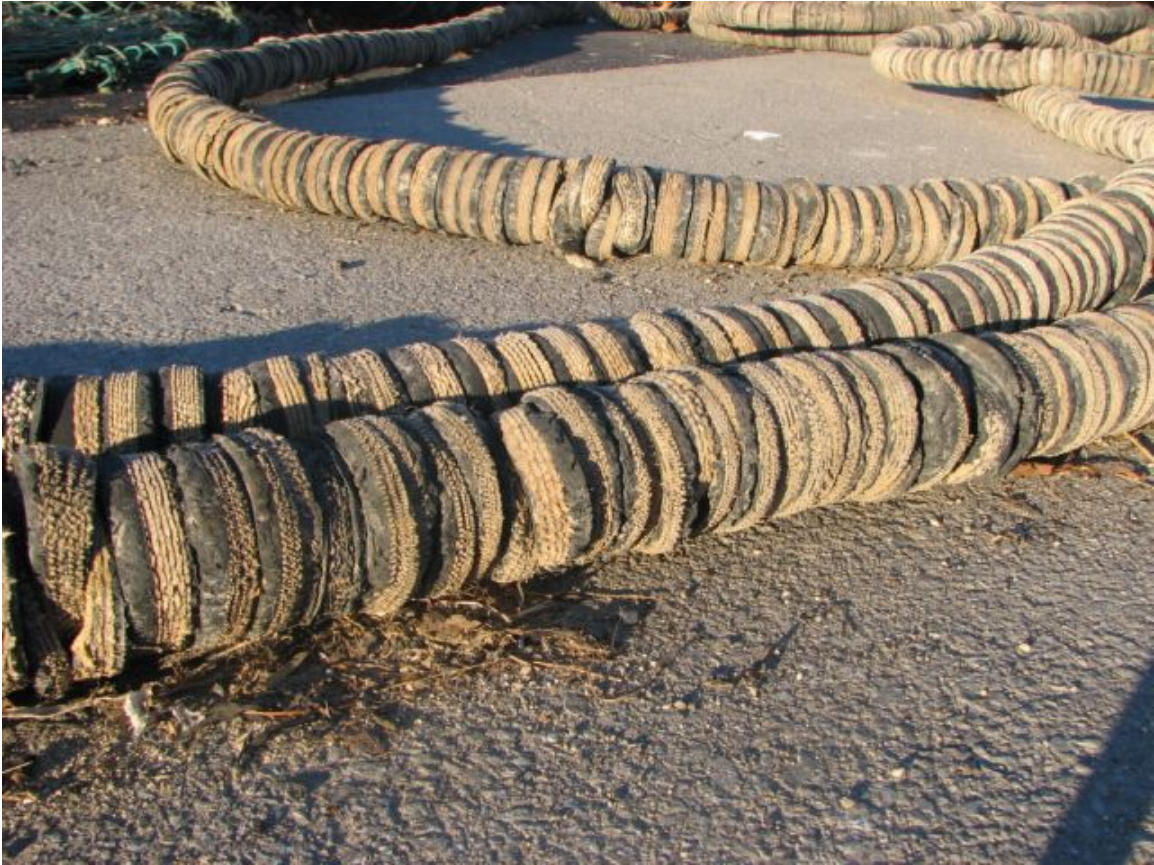
Figure 7 - Ground cable with cookies
